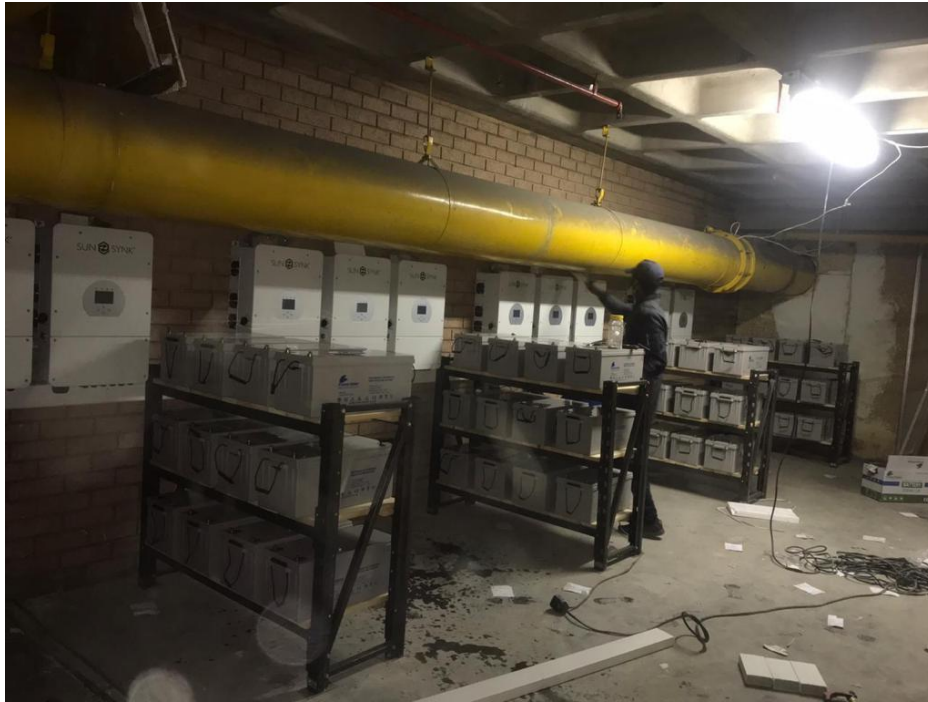
Figure 59 - Inverter installed in a dusty environment.
