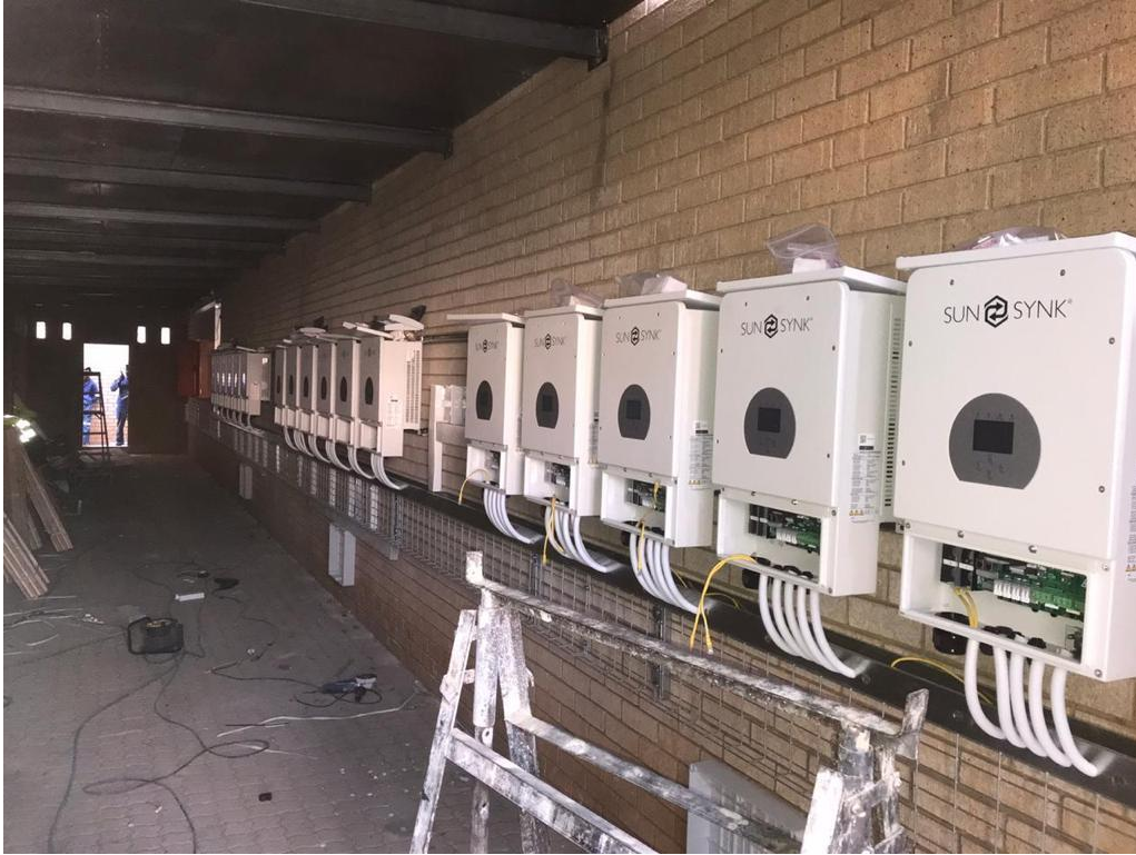
Figure 51 - Installation with many inverters.
