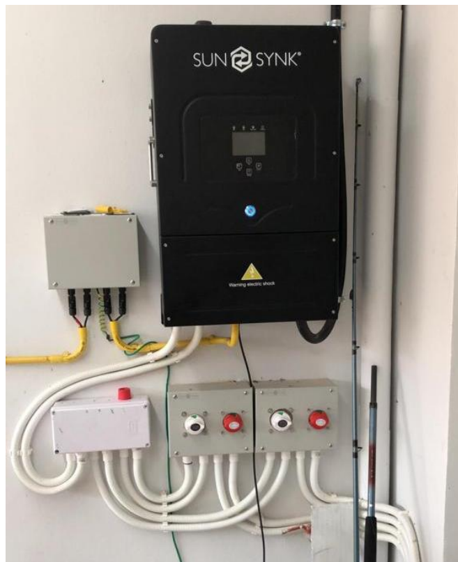
Figure 14 - Sunsynk inverter installation - black version.
