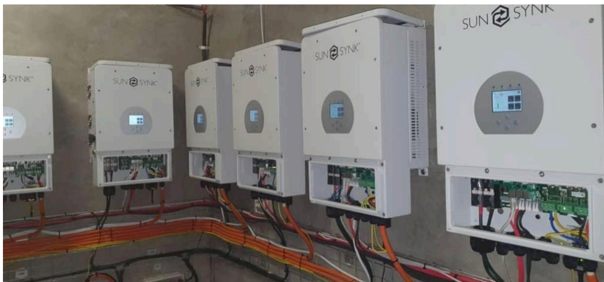
Figure 55 - Sunsynk inverters paralleled.
